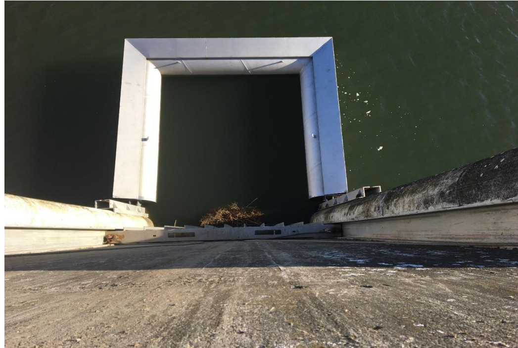
North exit debris guard in place. Trash rack raking required.
